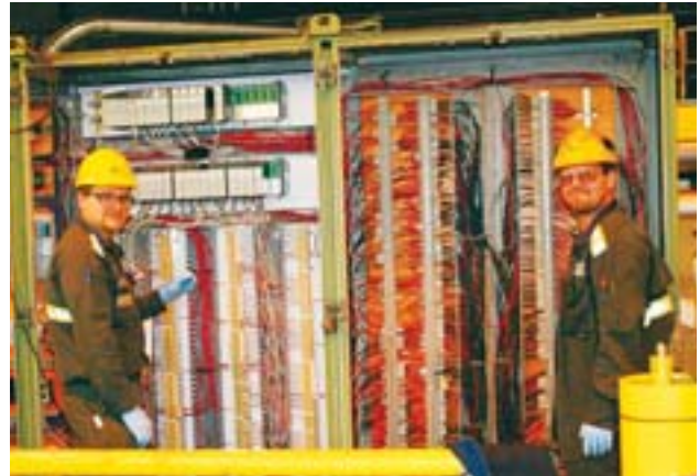
Apprentice electricians Aron Clement , left, and Braden Lamb worked on the new programmable logic controller (PLC) and harnesses. One can't imagine the thousands of meters of old wiring they pulled and new wiring they re-ran from the PLC to the motor control center (MMC).
