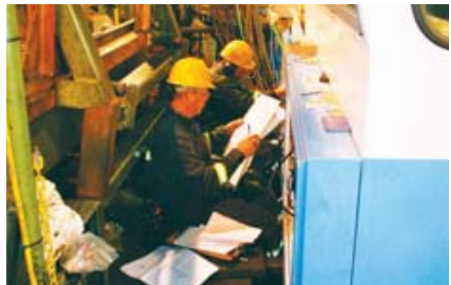
Electrician Duncan Peacock , foreground, and electrician apprentice Chad Stevenson work in extremely cramped and restricted quarters to first extract the old wires and control console and then install the new wires and control console.
