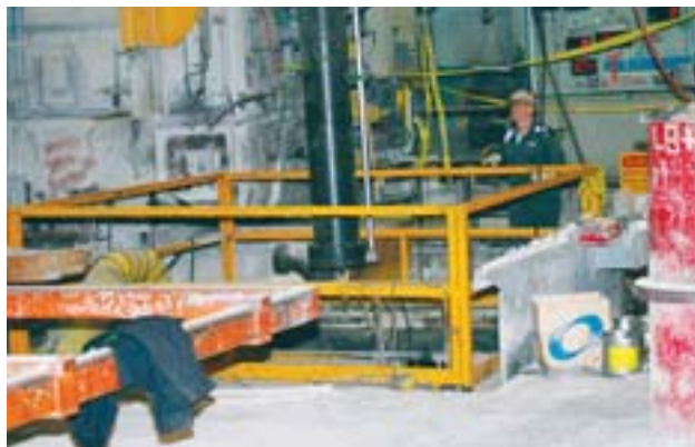
Millwrights Paul Quinn , pictured, and Rob Rowlett worked above ground directing the crane driver on placement to install the repaired 25-foot cylinder at DC-3. Meanwhile resources were also working 30-feet below in the pit to ensure the cylinder was positioned correctly.
