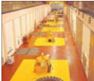
▲ Powerhouse in Kemano
