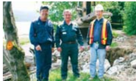
Dave Ringham, Mario Santos and Shawn Zettler take a break from erosion control.
