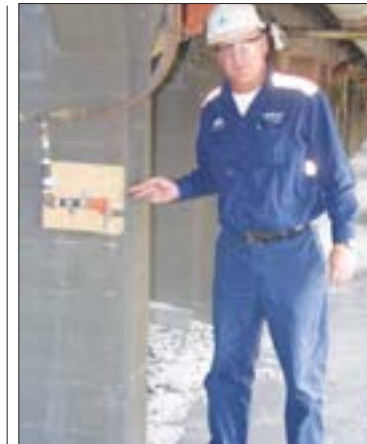
▲ In the line 5 potroom basement Scott Blackman points out one of the new air lines installed by the pipe shop crew.
