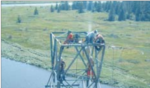
▲ BC Hydro crew pulls wire and does dead-end connection at the estuary tower. The first tower in the switchyard-T378 and the last in the estuary-T372 have dead-end connections on each circuit. The balance has suspension hardware installed on each tower and circuit. Photo Tracy Petley.
