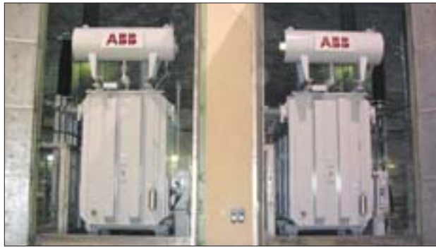
▲ Manufactured by ABB, these new state-of-the-art transformers should provide reliable service for years to come.
