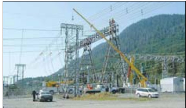
▲ Shown in the picture is the guarding on the buss and a hydro truck holding up a traveler to pull the wire along. BC Hydro crewmembers stand in the tower to monitor pulling and to do the dead-end connection. Out of site in the switchyard is the truck-mounted puller to pull in the second circuit. At other locations pole structures were installed to protect the A-area buss and the power lines on Eurocan's haul road and Alcan's dump and access road. Methanex allowed BC Hydro to shut down their line during pulling. Photo Tracy Petley.
